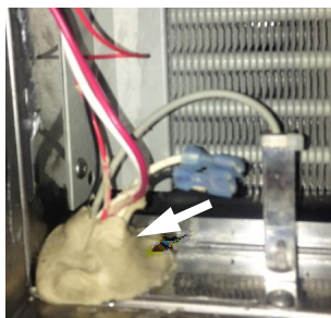
Figure 6-1. Sealing Compound at Wiring Pass-through
