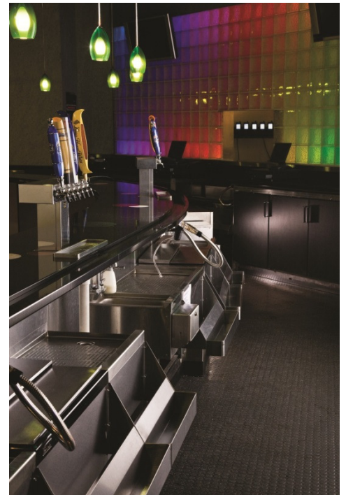
Perlick’s Top Shelf line of Stainless Steel underbar equipment installed at the Bradley Center in Milwaukee, Wis., includes pre-configured cocktail stations, drainboards, specialty sinks, corner filler sections, service stations and liquor displays.
